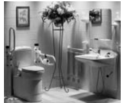
Fig. 16 Automated, height adjustable sinks and toilets accommodate a broad range of user abilities (photo from Linido USA)
