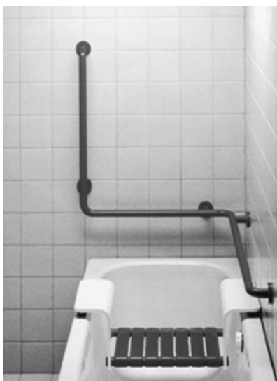
Fig.26 Grab bars installed in the bathtub area (photo by HEWI)
